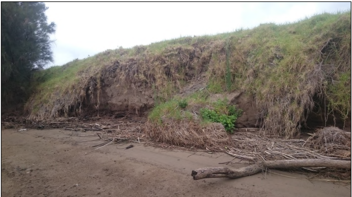
Figure 7. There was slumping of some section of river bank due to undercutting at the toe.
