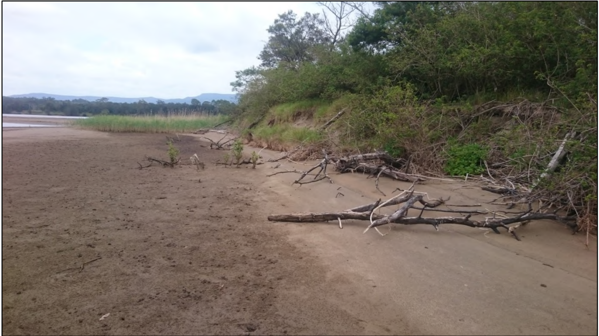
Figure 12. The western tip of the island is subjected to westerly wind chop at high tide. Sand sausage protection should be installed at the toe of the bank to slow erosion. There were also weeds such as Lantana camara that should be removed and replaced with Swamp Oaks.
